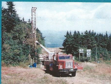
Top: Jack Frost and crew drill wells at Stratton summit (1968). Bottom: Frost drilling at the intersection of Polar and Black Bear trails (1981).
